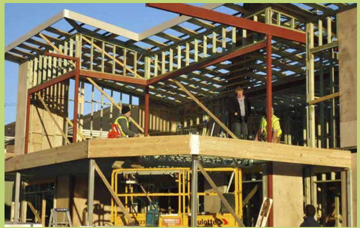
Putting in a fantastic team effort from AA & KA Jones Builders were Trent Riddle, Nick Sherlock and Kedar Giles, pictured with Charity House Co-Project Manager, Rod Papworth
